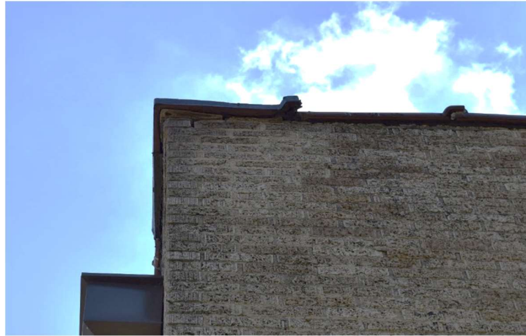
Figure 5.14: Coping tiles lifting up in the northwest corner due to damaged parapet. Lifting and displacement likely caused by corrosion of metal built into wall assembly.
