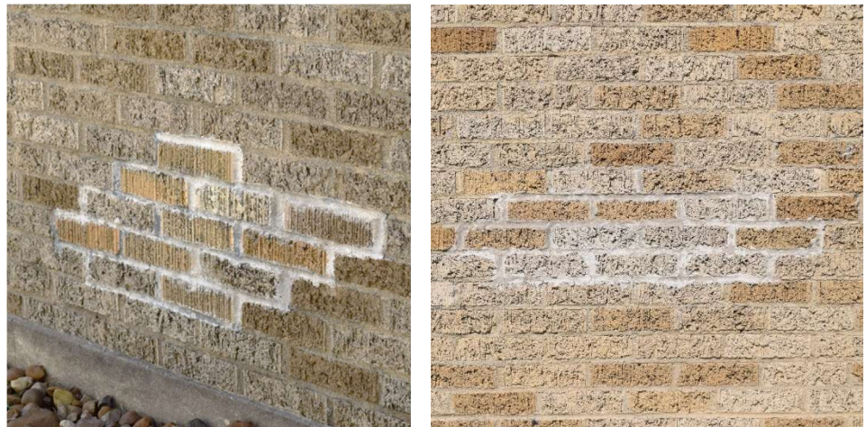
Figures 5.18 and 5.19: New bricks at the north wall (left) and relocated bricks on the east wall (right) taken from that location on the north wall.
