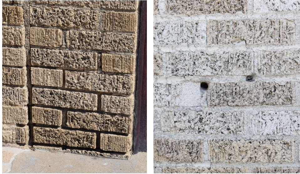
Figures 5.20 and 5.21: Deteriorated mortar in need of repointing. Anchor holes in the masonry on the west façade.
