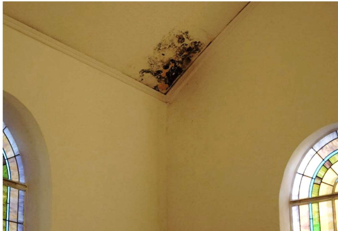
Figure 5.27: Water damage to ceiling and walls in northwest corner (northeast corner exhibiting similar damage).
