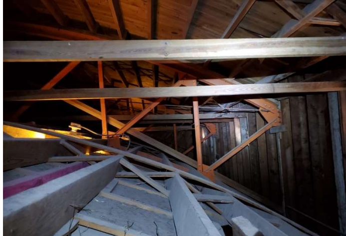
Figure 5.26: Steel truss and ceiling framing in good condition where observed, viewed from the southeast corner.
