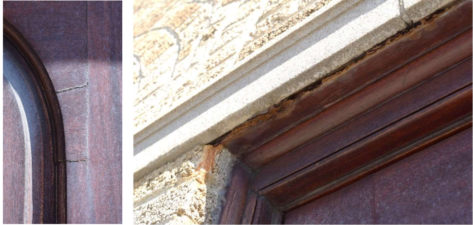
Figures 5.24 and 5.25: Cracked panels on the front door with no protective coating. Oxidizing steel lintel above the front doors jacking the masonry above upwards and outwards.
