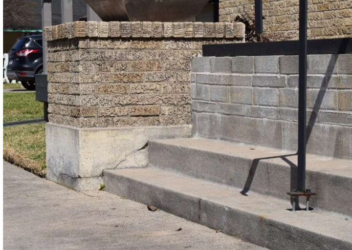
Figure 5.08: Cracks visible on the front stair cheek wall foundations.
