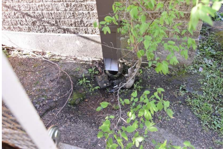
Figure 5.15: Downspout at the northwest corner of the building discharging partially into subgrade drainage but also directly onto the soil next to the foundation.
