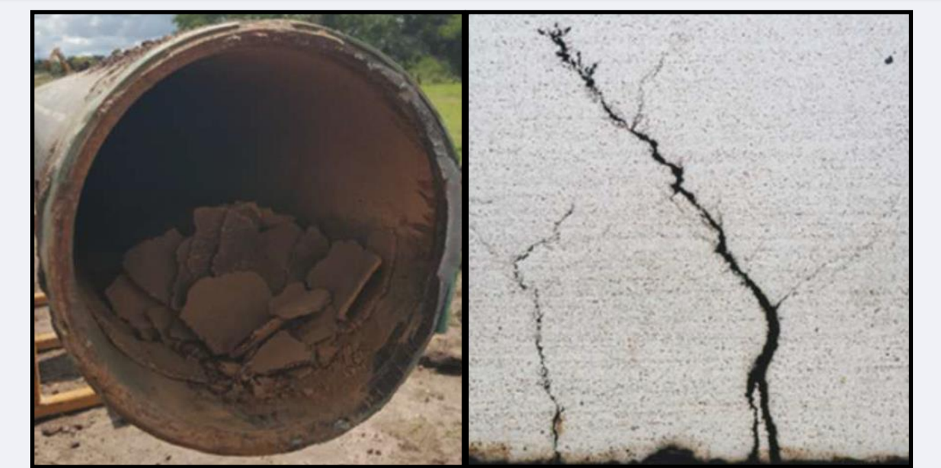
Figure 1. SCC failure in presence of amine-based H 2 S scavengers
